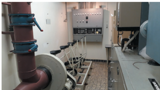
Oostburg, commandopost, luchtbehandelingskamer BB commandopost (foto Henk Hendrikse)
